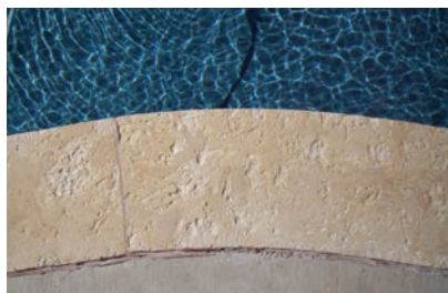
Salt spalling on travertine around a saltwater pool
